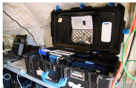
Edge Connect is set up on site at Palau International Airport during Valiant Shield 22. (U.S. Air Force photo by Senior Airman Jose Miguel T. Tamondong)
